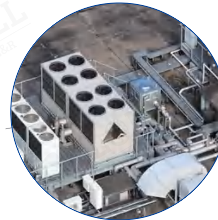
Building Ventilation System
