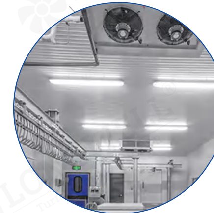
Workshop Ventilation System
